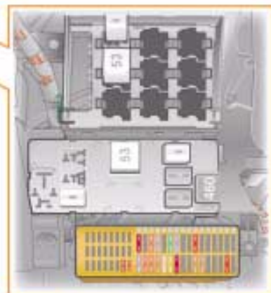
Fuse box on left under dash panel
