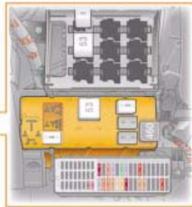
Relay carrier on control unit for onboard supply, on left under dash panel
